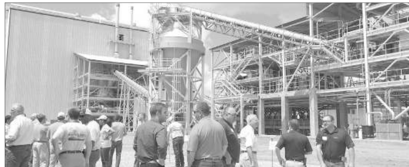
Guests at Monday's event line up for tours of the new, multi-million dollar mineral sand processing plant.
